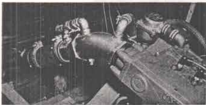
Fig. 8 Photo of Exhaust Piping
